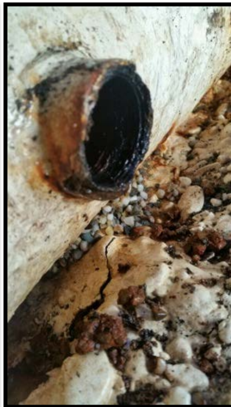
Rusted effluent manifold couplings
