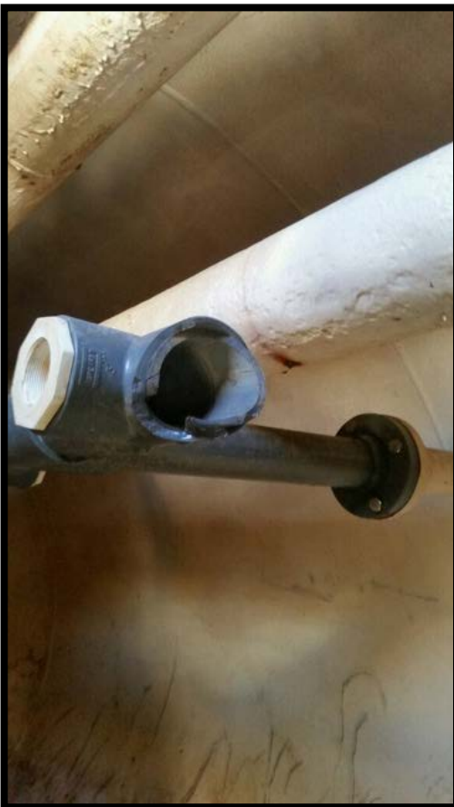
Broken Surface Wash Piping
