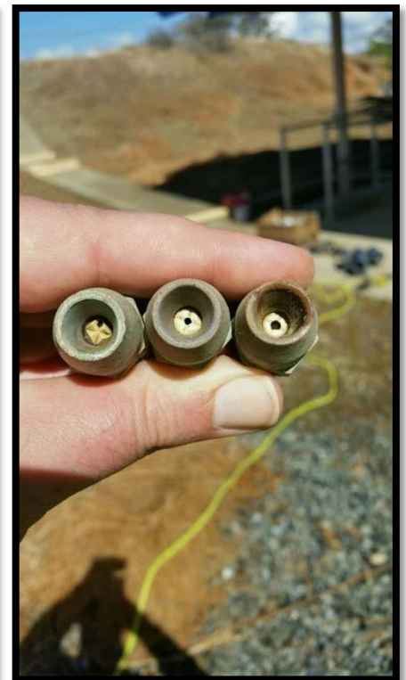
Clogged Surface Wash Nozzles
