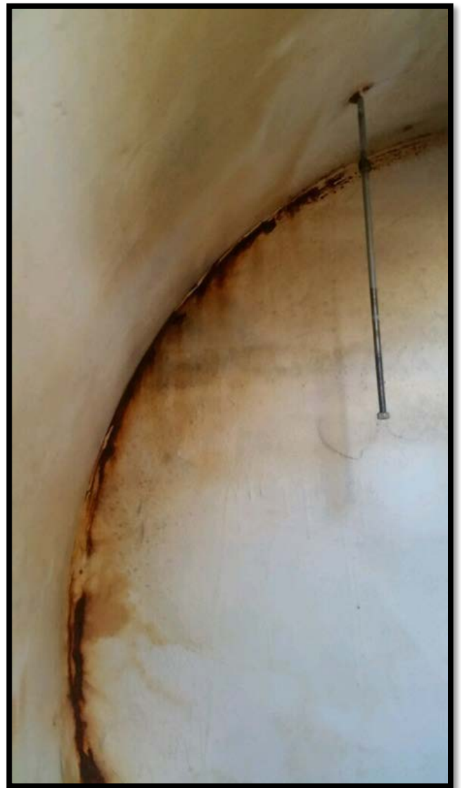
Corrosion, Holes and missing Coatings at Bulkhead
